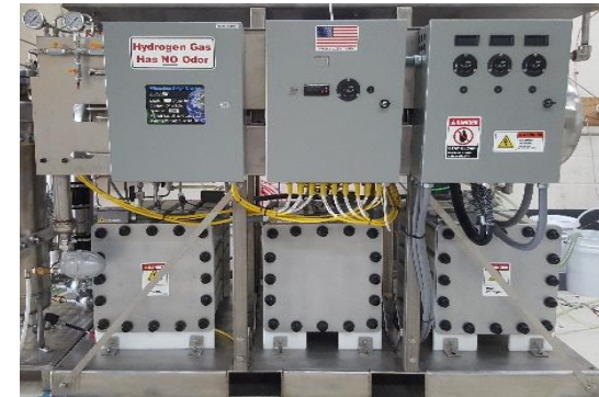
3 stacks Pumped water circulation
