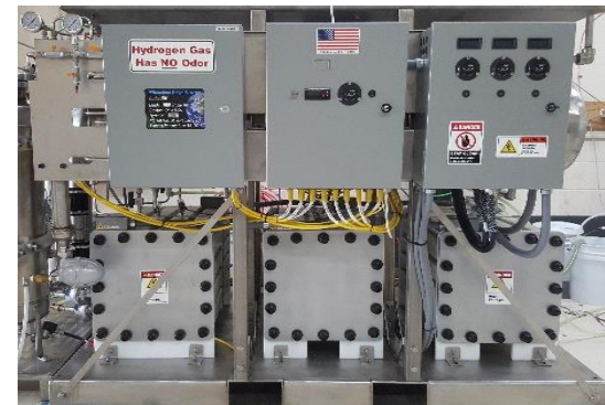
3 stacks Pumped water circulation
