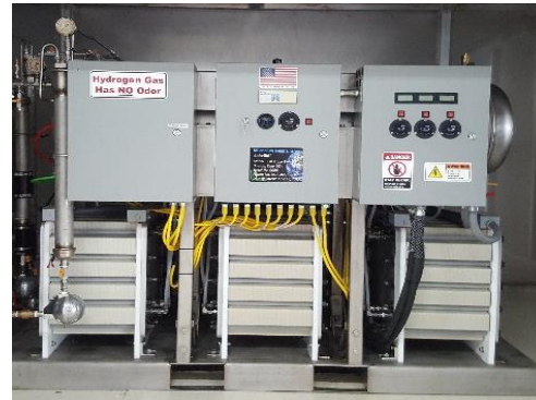
6 stacks Passive water circulation
